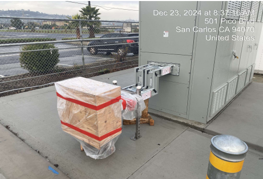
the bus duct was installed and staged for the PGE power cutover
