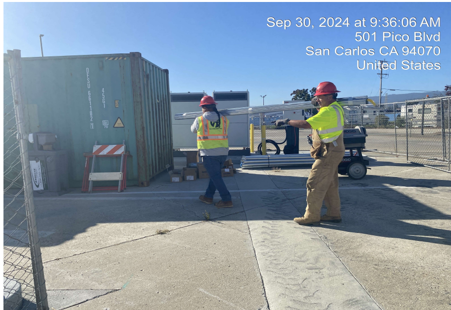
Anvil Power received materials and prepared to install the conduit between MDPO-1 and Building 700.
