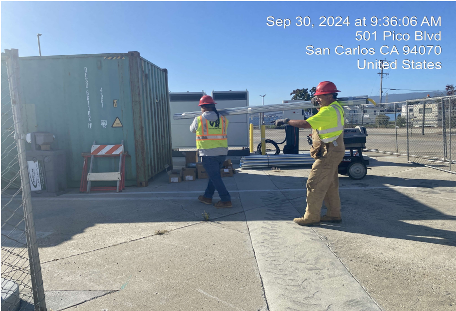
Anvil Power received materials and prepared to install the conduit between MDPO-1 and Building 700.
