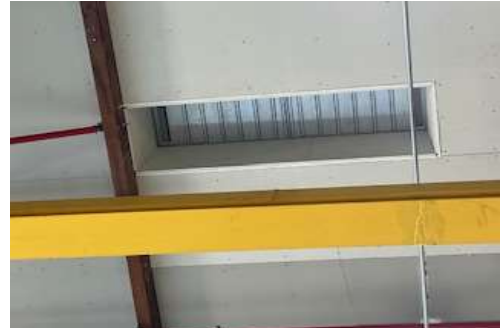
Refinement of the exhaust duct (NB Building 100)
