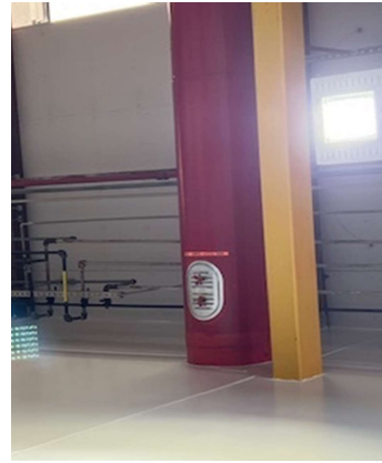
Fire Damper Door installed (NB Building 100)
