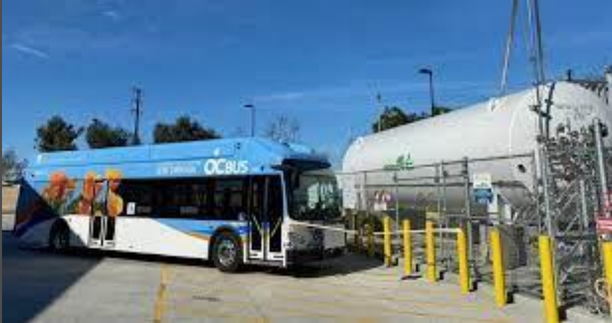
Hydrogen Storage & Fueling Station
