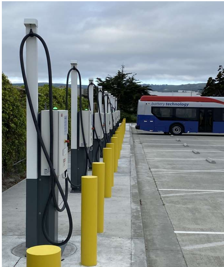
North Base BEB Interim Chargers
